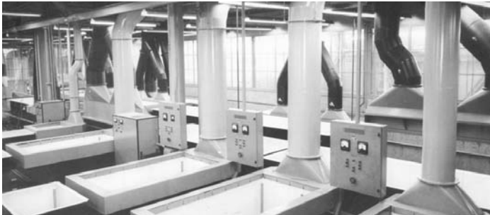
Welded Thermoplastic Hoods, Ductwork and Tank Liners In Large Plating Operation
